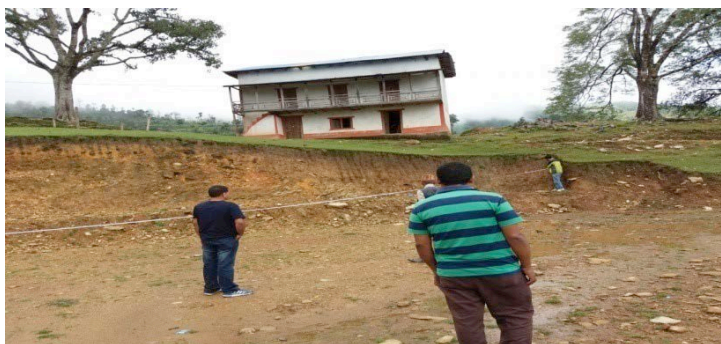
Figure 3: (Land is being measured at the site for CRC building at Nagdaha, Ramechhap)
